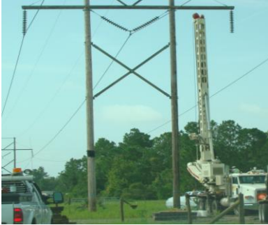
Figure 2: Existing 230 kV transmission line with H Frame structure.
