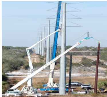
Figure 4: Single pick robotic arm which captured the energized conductor above the H frame structure.
